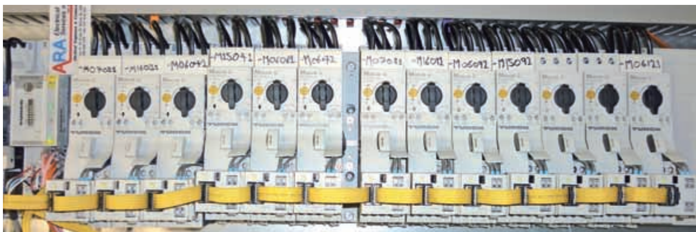
The motor starters, which are connected with a BL20 DeviceNet gateway, are installed in no time at all
