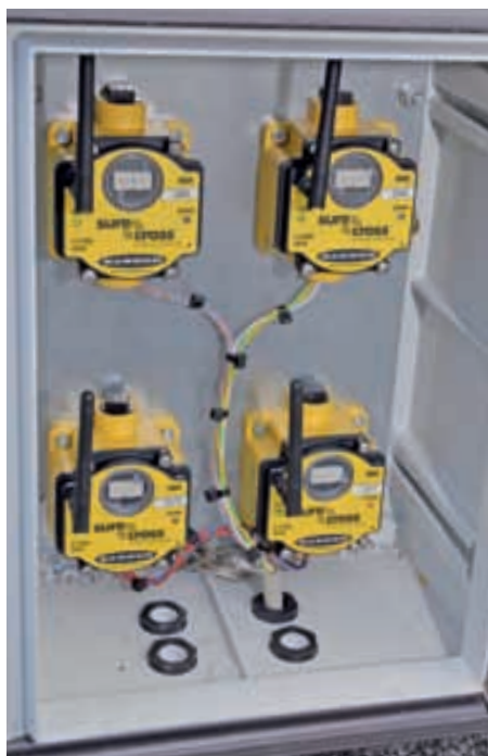
On the roof of the station, four radio receivers are installed
