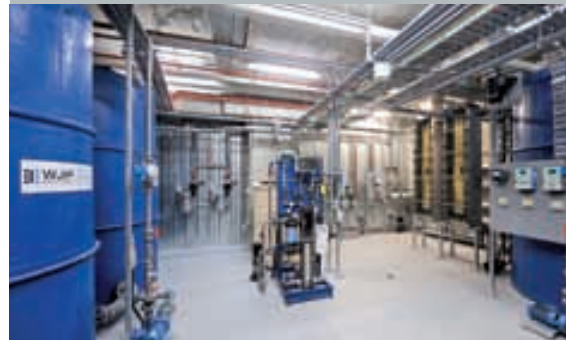
In Australia, WJP Solutions uses Turck's robust connection technology and BL20 distributed I/O system for their modular water treatment plants. Page 32
