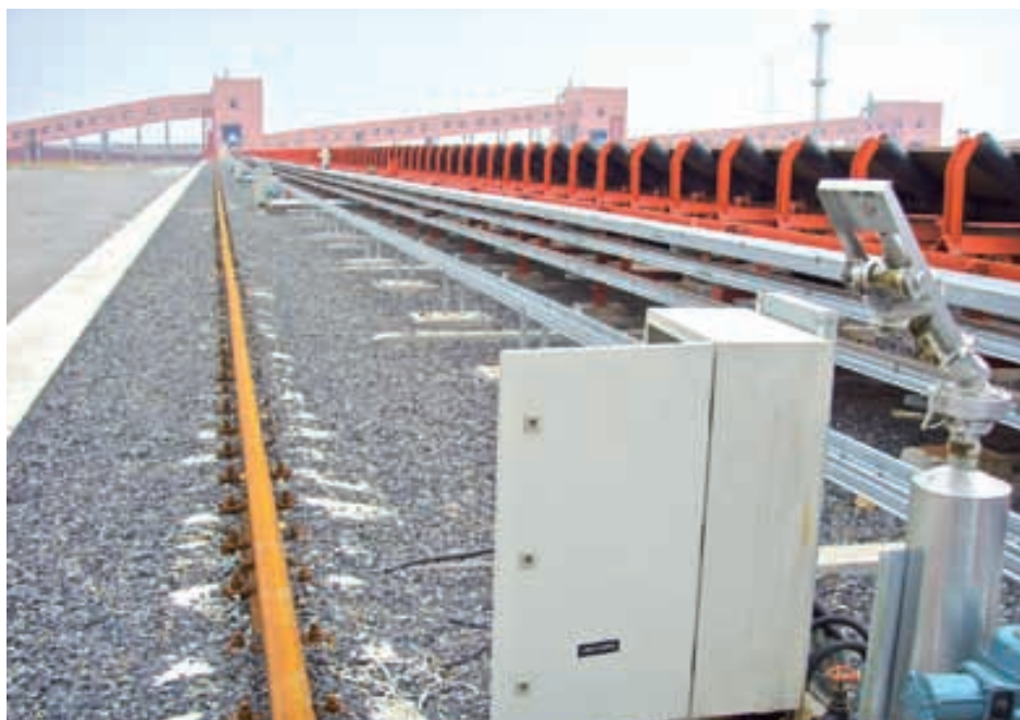
Each sprinkler is equipped with a control cabinet with a BL20 station
